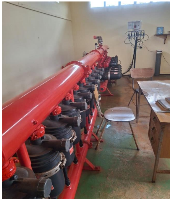
Photo 1 – View of the existing spin-Klin Filter Units of Solitude II Filtration Plant
